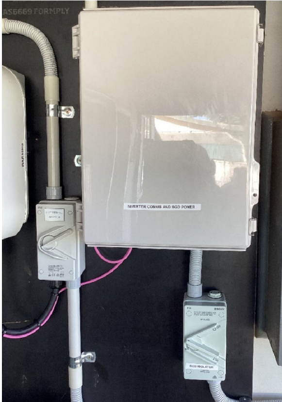
Figure 5: Example SGD installation
