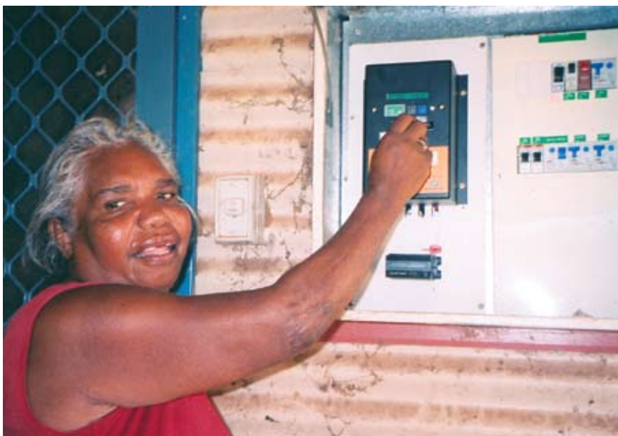
Nulleywah resident, Emily Hester is one of ready power's first customers.
