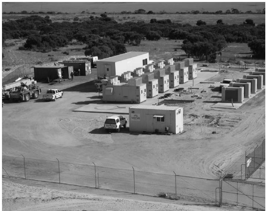
▲ Overview of the new Hopetoun Low Load Diesel Power Station.
