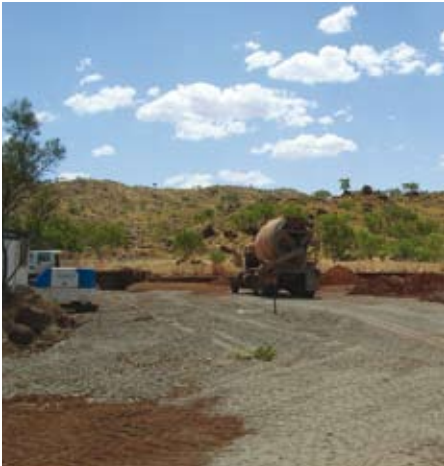
▲ Civil works are under way for the new power station at Warmun.
